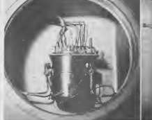
HYDROGEN ANALYZER along with sampling apparatus are among fastest analyzers installed at Lago. Installed at PCAR, it gives a reading every minute by correlating temperatures with hydrogen content.
